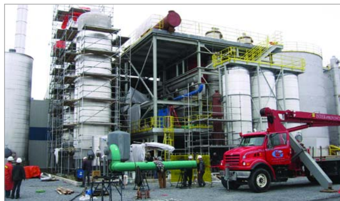
GreenField Ethanol's Quebec ethanol plant, shown here under construction in 2006, held a tour for the 2007 Alcohol School.
